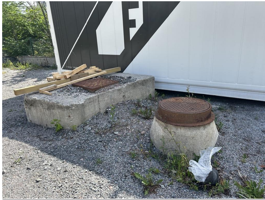
Figure 4: Inspection well connected to Stockholm City's main sewer system
